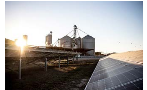
Installed Solar Panels
