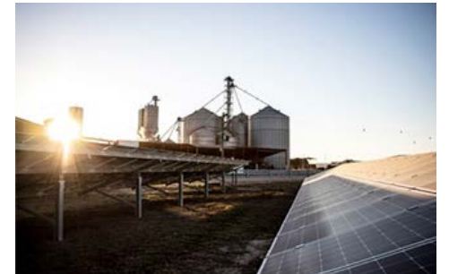
Installed Solar Panels
