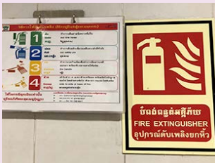
All Signs in Cambodian on Fire Prevention Facilities
