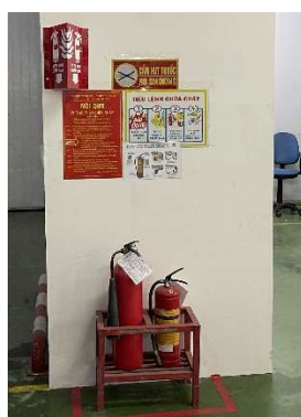
(Center) Easy-to-understand installation of fire extinguishing equipment
