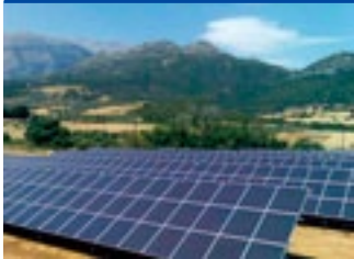
Distomo solar park in Greece
