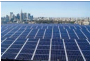
Solar panels on the roof of our Tokyo headquarters building
