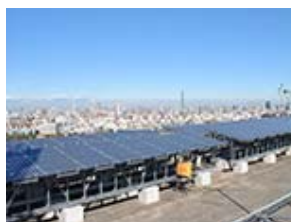
The solar panel installed on the roof of ITOCHU Corporation's Tokyo Head Office building
