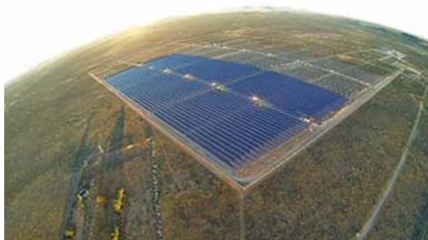
The 75-MW solar power generating system selected in the first bid, currently under construction
