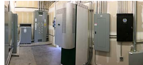
Green Charge Energy Storage
