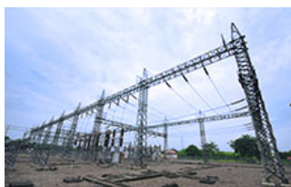
Power substation for KIIC
