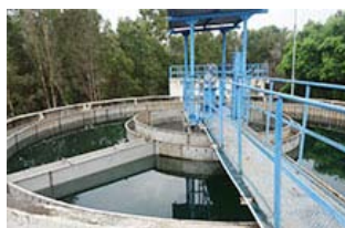
Water treatment facility that meets the government standards of Indonesia
