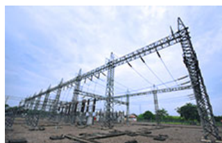
Power substation for KIIC
