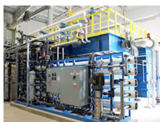
In-house water waste treatment facility
