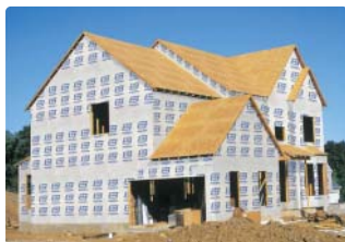
Home construction site in North America; materials supplied by PrimeSource Building Products, Inc., and other companies
