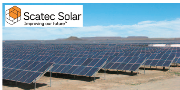
The Kalkbuit photovoltaic power generation facility, one of the largest in South Africa
