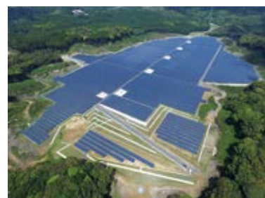
Saga-Ouchi Solar Power Station, Japan
