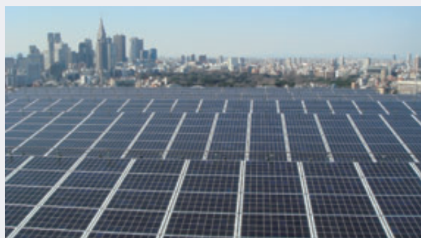
Solar Business Department: Solar power generation plant at the Tokyo Headquarters of ITOCHU Corporation
