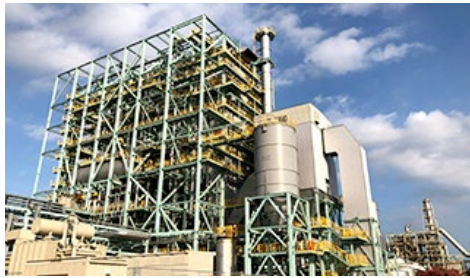
Ichihara Biomass Power Plant
