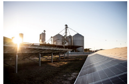
Installed Solar Panels
