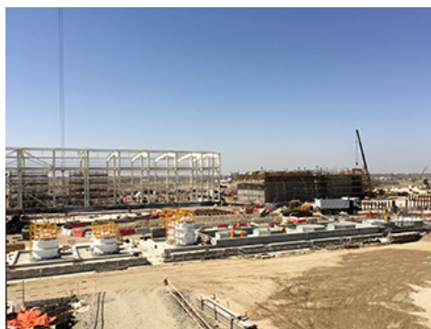
Seawater Desalination Plant
