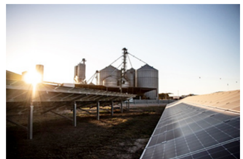
Installed Solar Panels
