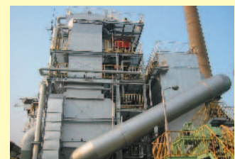
Biomass-fueled boiler equipment
