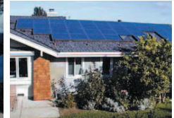
Solar cells installed on the roof of a home
