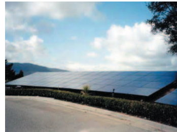
Large solar cell installations for residential use
