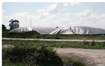
"Covered lagoon" equipment installed at a waste treatment facility captures methane gas produced through fermentation
