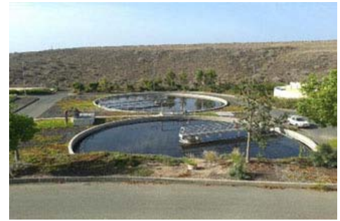
Waste water treatment plant - Gran Canaria
