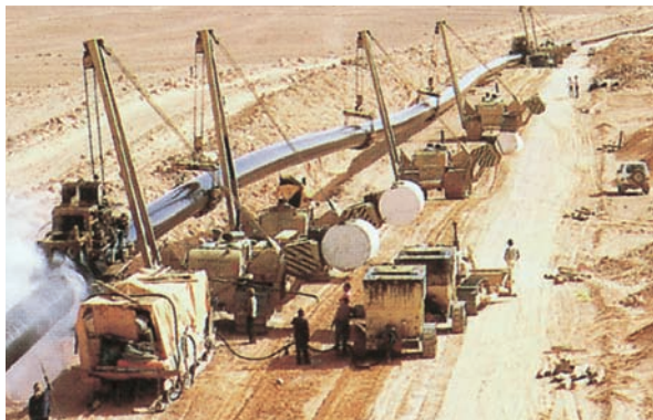
A natural gas pipeline in Algeria
