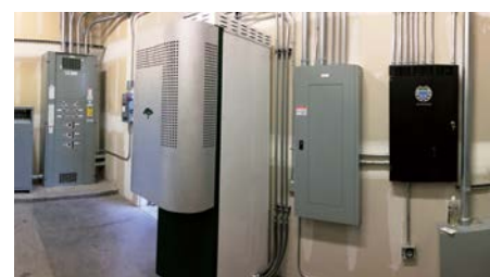
GCN's storage battery system in use at a university in California
