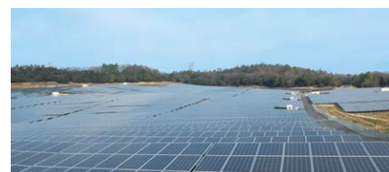
Shin-Okayama Solar Power Plant (commenced commercial operation in January 2017)
