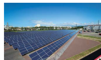
Solar panels installed on unused land at the Mikuni factory
