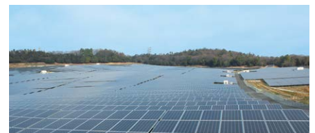
Shin-Okayama Solar Power Plant (commenced commercial operation in January 2017)
