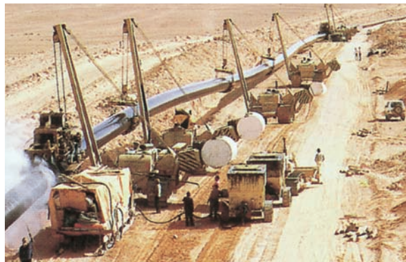
A natural gas pipeline in Algeria
