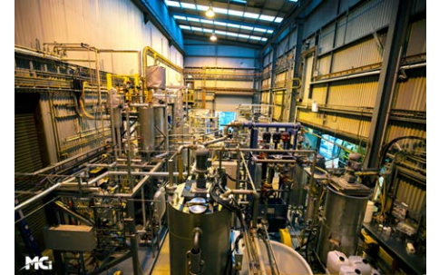
MCI's Pilot Plant in Newcastle, Australia
