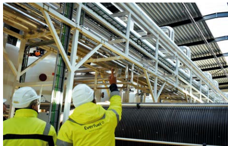
Inside the Plant
