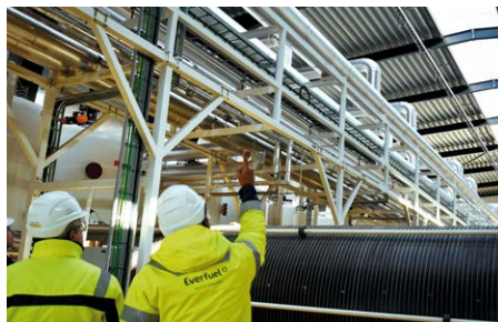
Inside the plant
