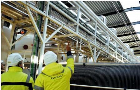
Inside the plant
