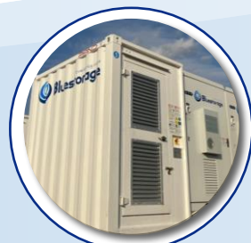
Power & storage plants
