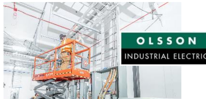
Electrical Equipment and Construction Services
