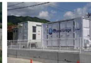
Grid-scale battery storage
